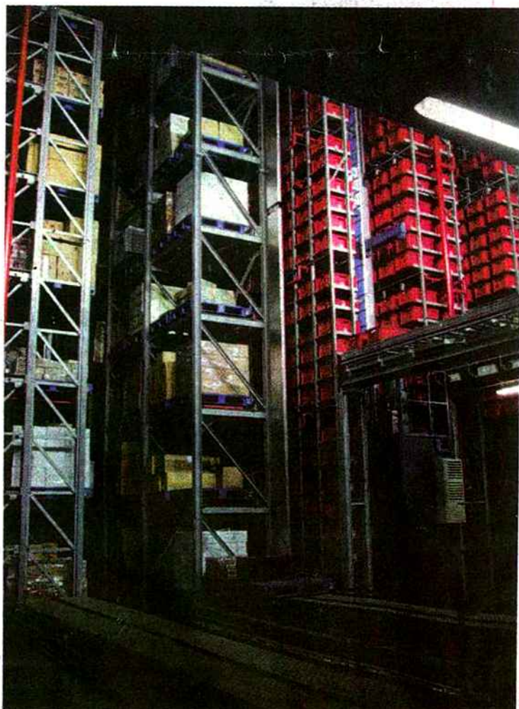
SECRET OF SUCCESS. This high-bay retrieval and storage system ensures automated, fast and efficient inventory and movement of goods and equipment from floor to floor of the huge CPCS building.
