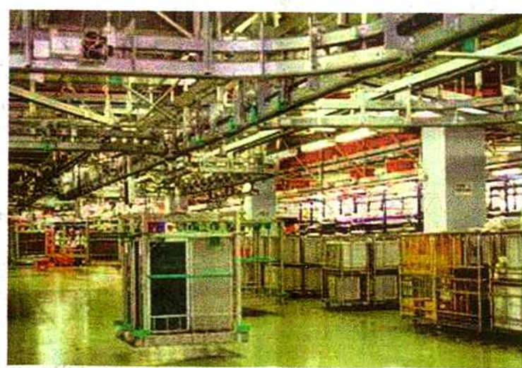
INBOUND area has a state-of-the-art conveyor system.
